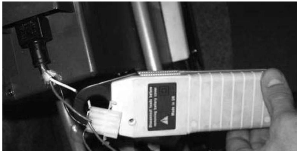
Figure 4.7: Current Measuring Device Clamped on the Battery's Hot Wire
